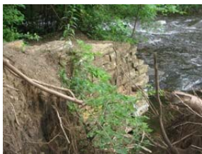
Eroding bank slope and failing wall.
