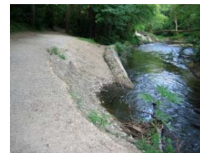
Failed wall and eroding bank slope.
