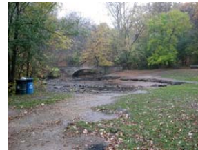
Stream velocity during heavy rainfall events has eroded the stream bank. Garbage cans would likely be swept away in a spring rainfall event without restoration work in this area.
