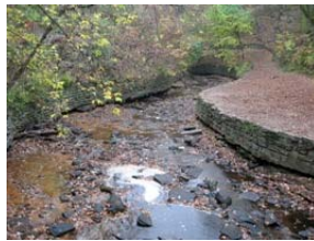
Temporary techniques preventing the crib walls from failing. Walls have been undercut due to stream velocity during heavy rainfall events. Walls will receive new footings during restoration work.
