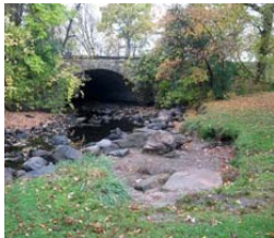
Stream velocity during heavy rainfall events has eroded the stream bank.
